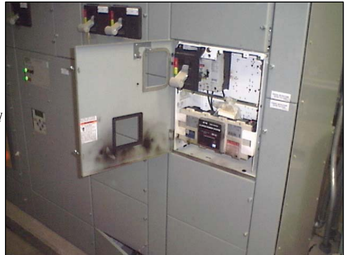
Switchgear Collateral Damage Due to Failed, Integral SPD Device
